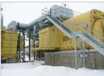
MH Synchronous Condenser
