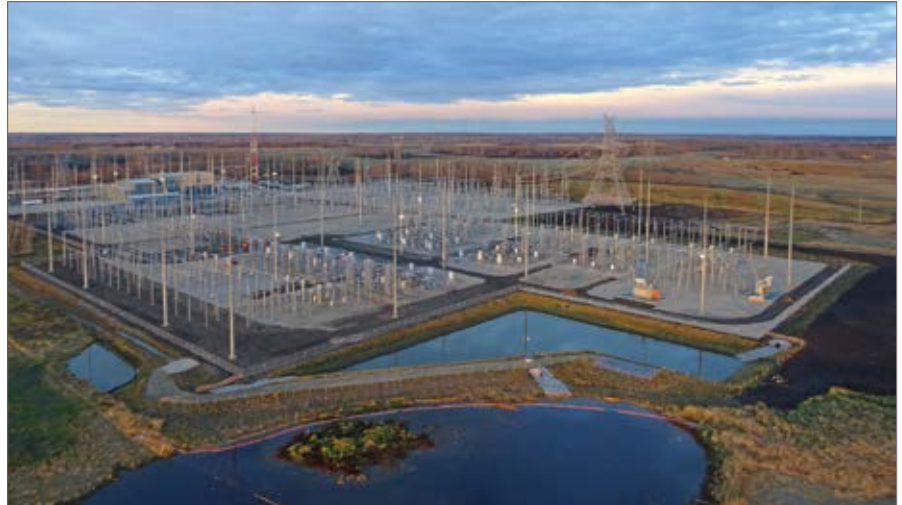
AltaLink WATL Sunnybrook Converter Station
